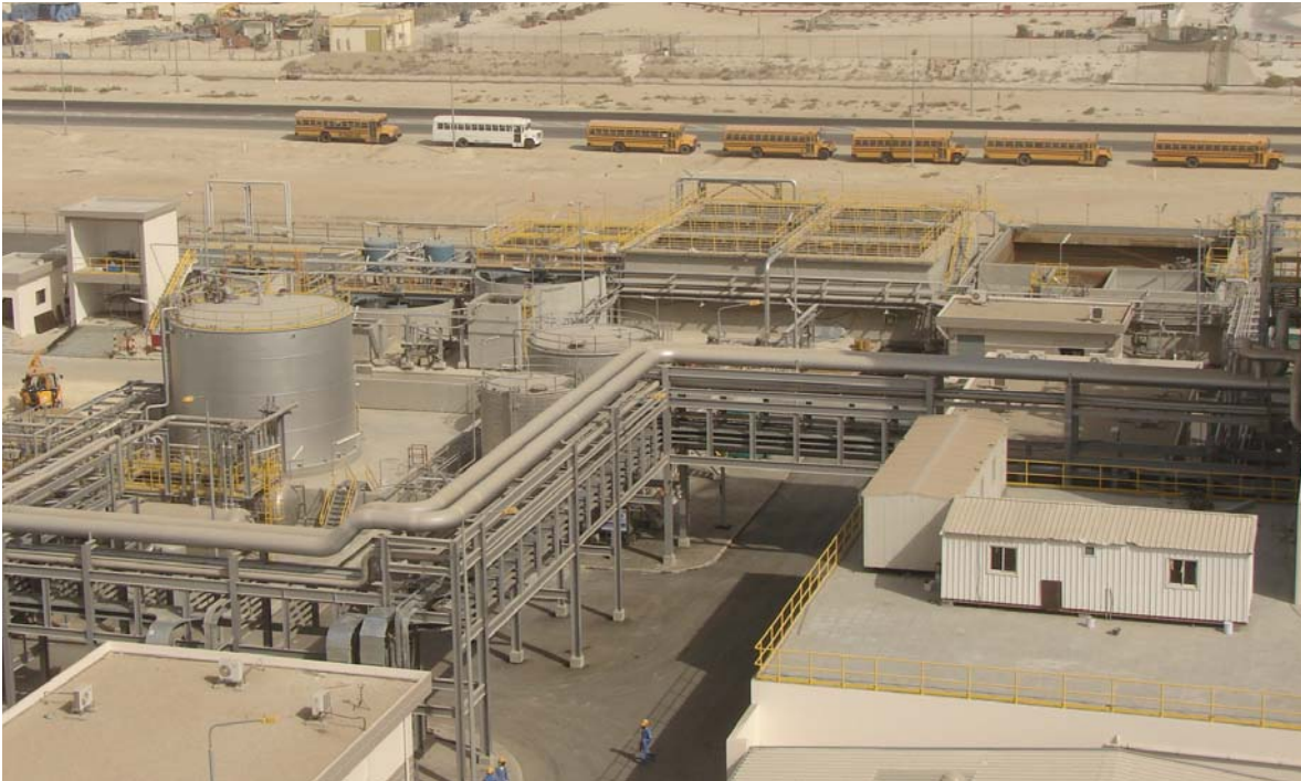
Chemanol – Saudi Arabia , Effluent Treatment Plant.
